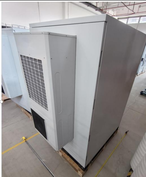
Photo 2 可充电锂离子电池能量存储系统背面 Back view of Rechargeable lithium-ion battery energy storage system
