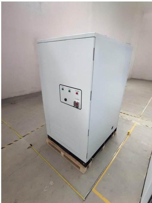
Photo 1 可充电锂离子电池能量存储系统正面 Front view of Rechargeable lithium-ion battery energy storage system
