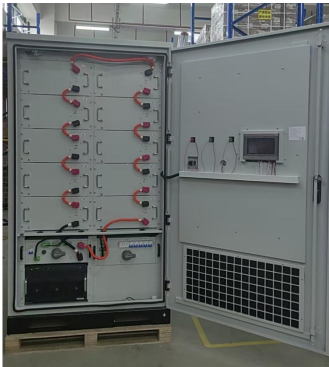
Photo 4 可充电锂离子电池能量存储系统内部图 Interior view of Rechargeable lithium-ion battery energy storage system
